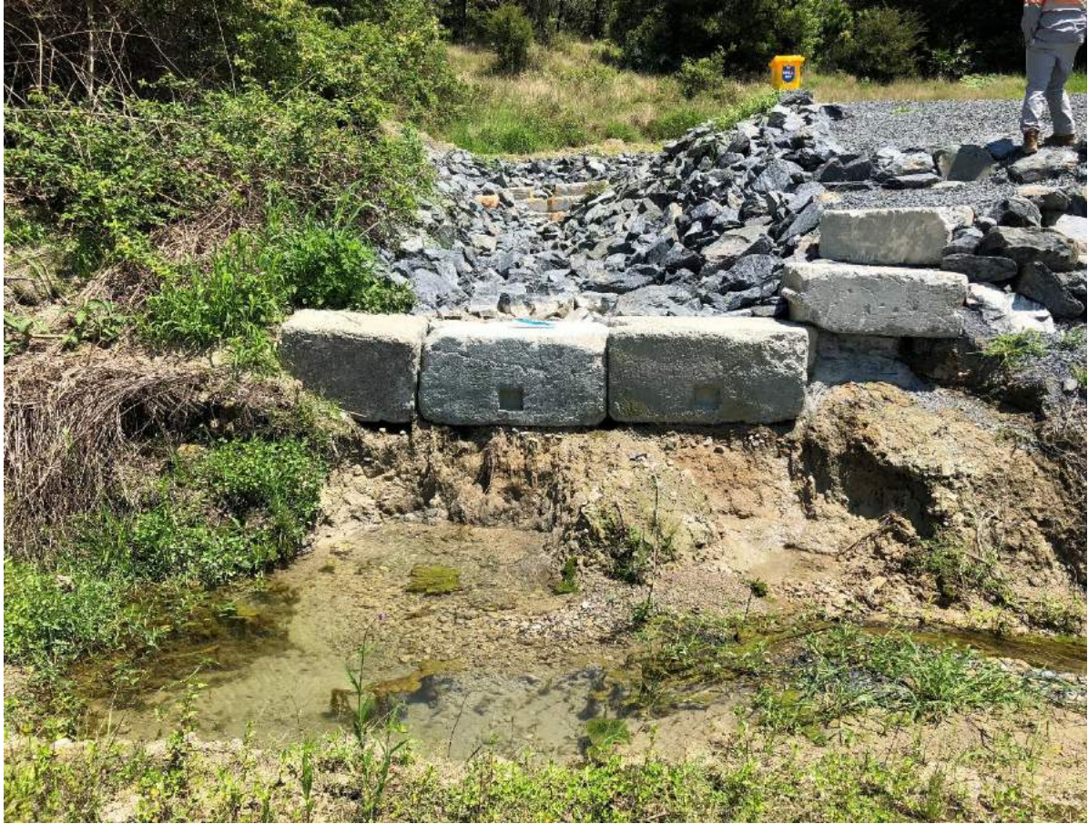
Photograph 7: concrete block weir located at the LDP at Site boundary, corresponding to Water Monitoring Location #2
