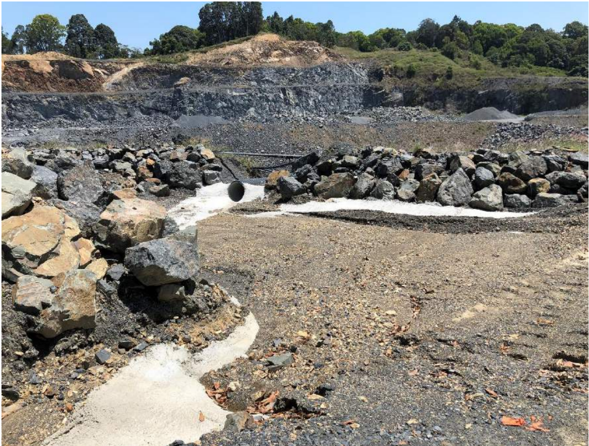
Photograph 18: Concrete lining of catch drains along upper access road
