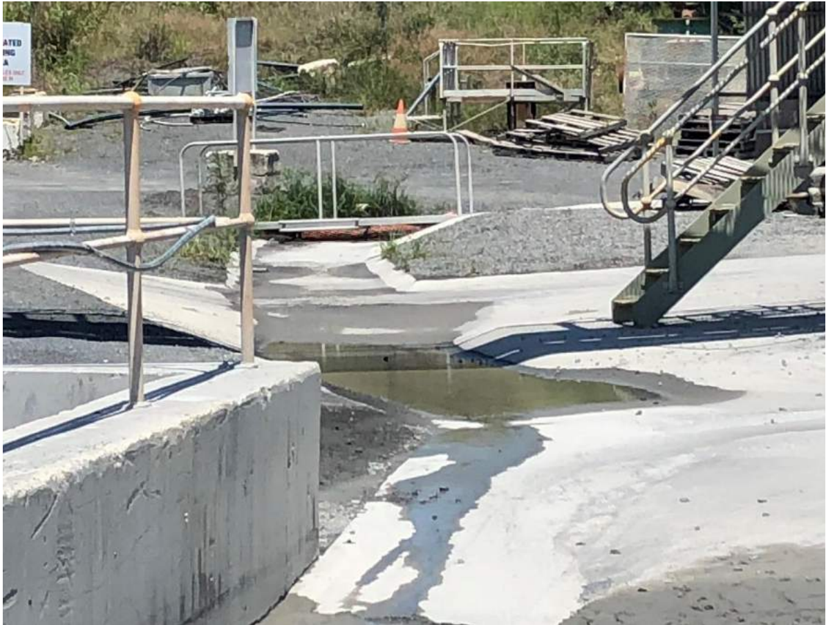
Photograph 11: Concrete lined drains draining to wedge pits
